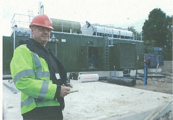
Checking the gas engine operation
